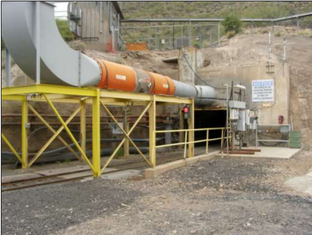
Entrance to Never Sweat Tunnel with ventilation system (June 2015)
