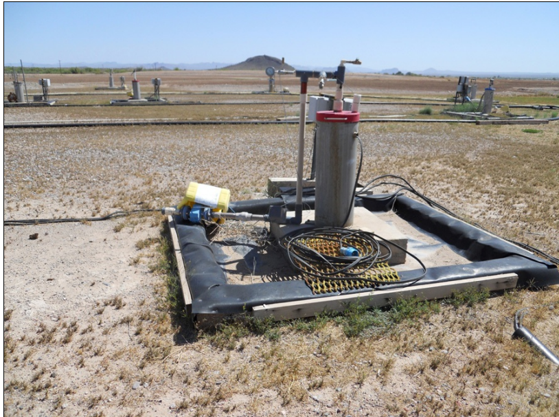
In-situ Leach Well Field at Florence Copper Project, Pinal County, Arizona (Photo taken by Jan Rasmussen, April 2012)
